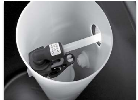
Connection at Brine Safety Float in brine tank
