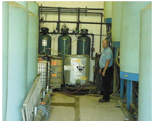
Chester Biadasz, president of Beaver of Wisconsin, visits the water treatment room at N&M Transfer, Neenah, Wisconsin. Storage tanks of treated water and waste-water surround him.
